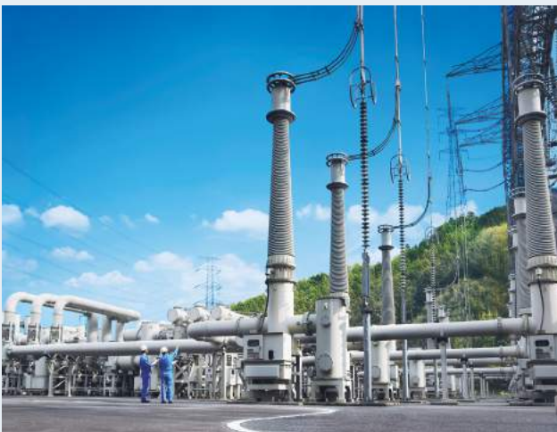
Mitsubishi Electric Transmission and Distribution Systems Center
