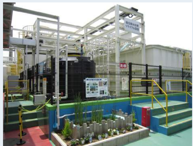
Water recycling equipment for the new metal plating process
