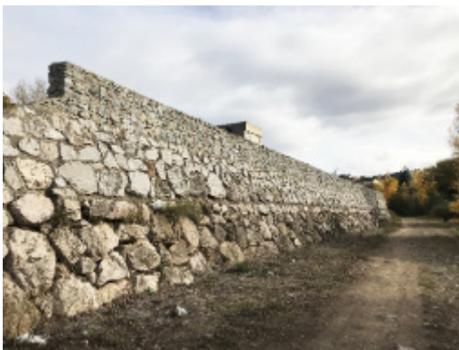
Raised 200 m-long wall at the confluence of two rivers where floods had occurred in the past (Spain)
