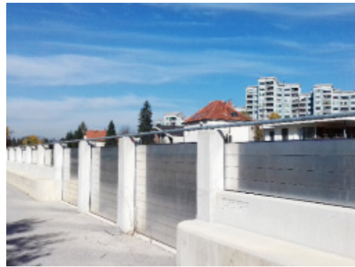
River dike with removable walls allowing the controlled flooding of one river bank, in order to protect the opposite densely populated bank (Slovenia)
